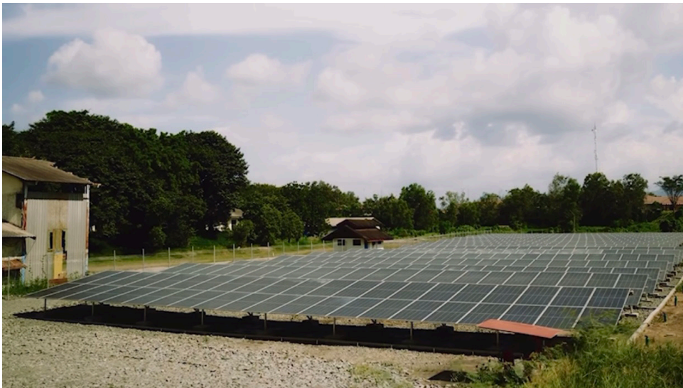
Smart PV project for a mining area in Indonesia
