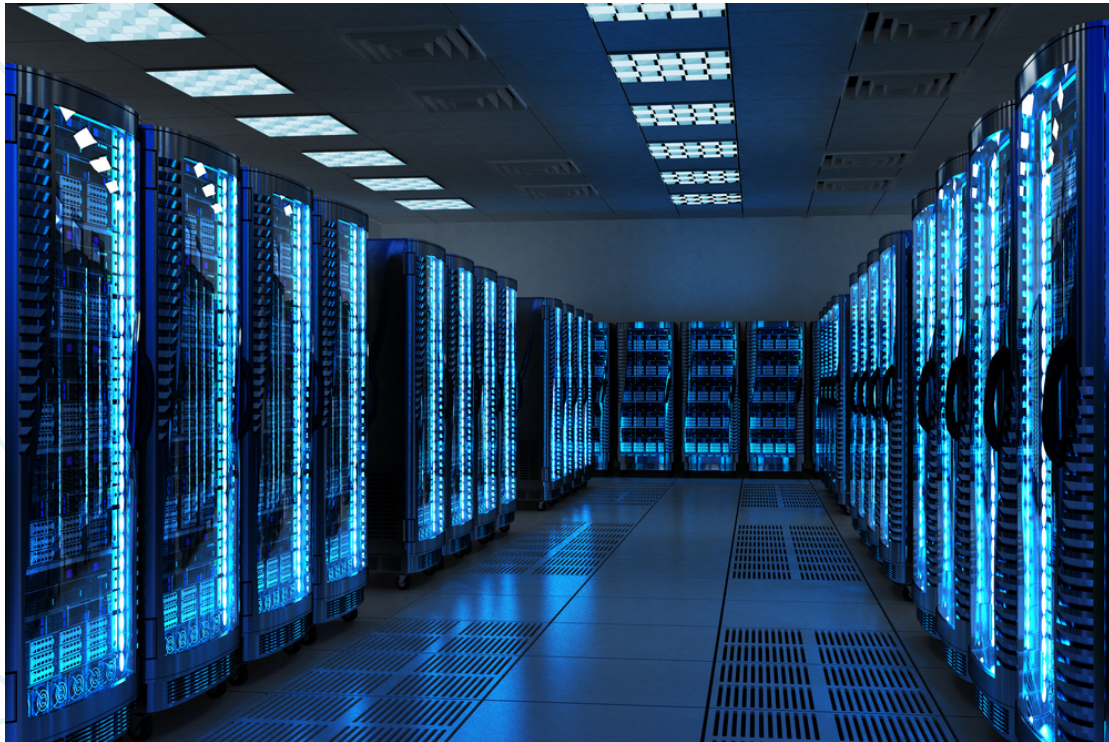
Figure 1.4. Data Center in the Intelligent Computing Era
