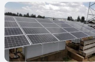
Site | Equipment room | Data center
