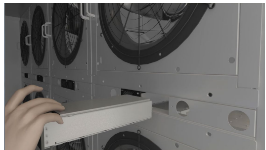
Plug-in maintenance on fan driver
