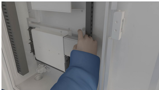
Plug-in maintenance on controller
